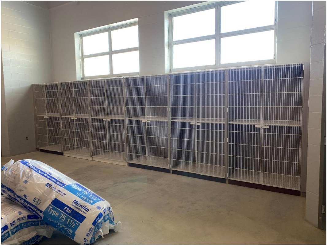
Instrument locker are installed.
