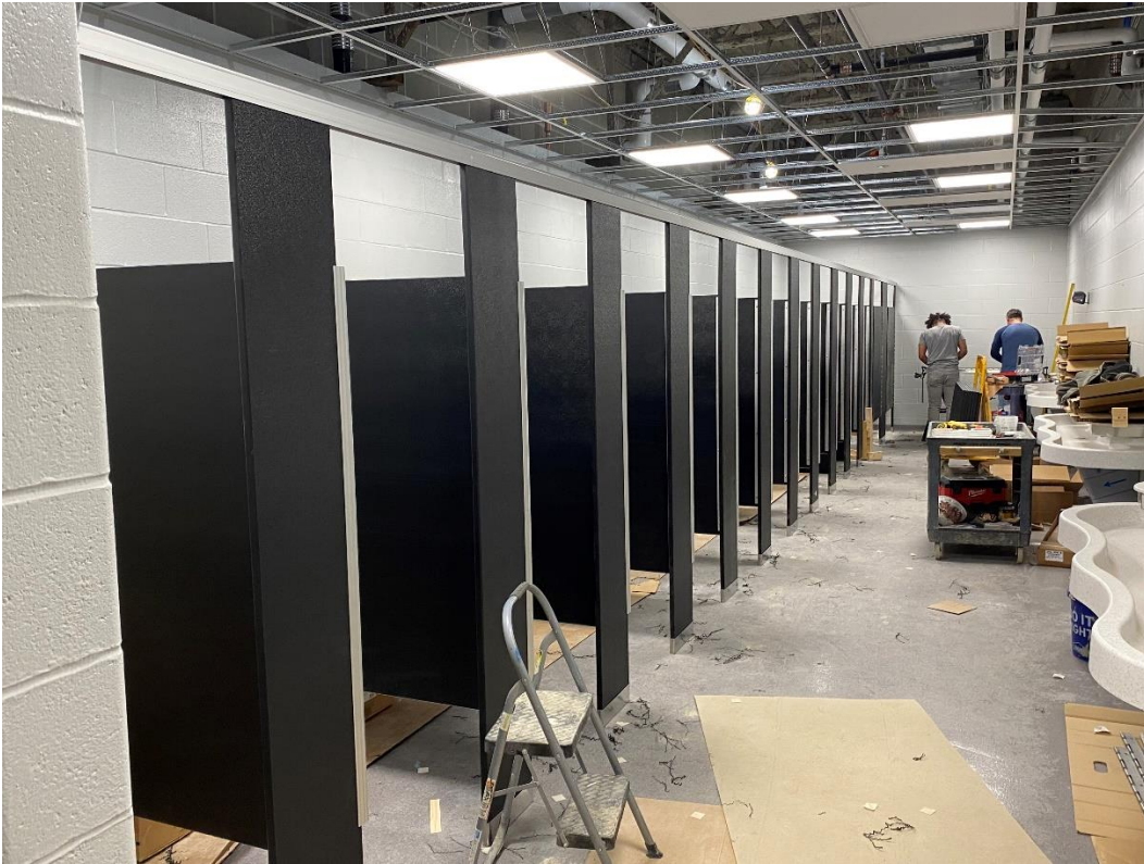
Toilet partitions in the main toilet rooms east of the Gym are nearly complete.
