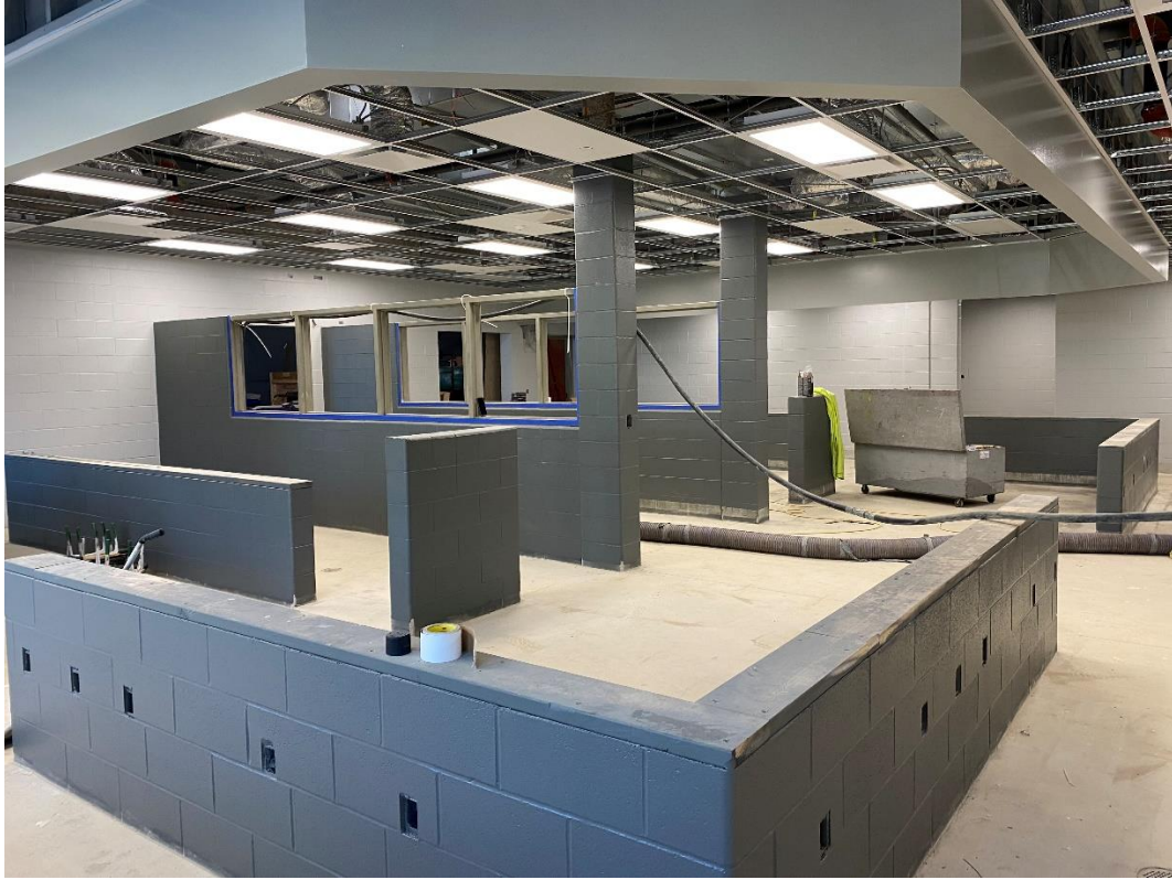
Ceiling grid is installed and walls are painted in the Kitchen. Floor finish will be installed this week.
