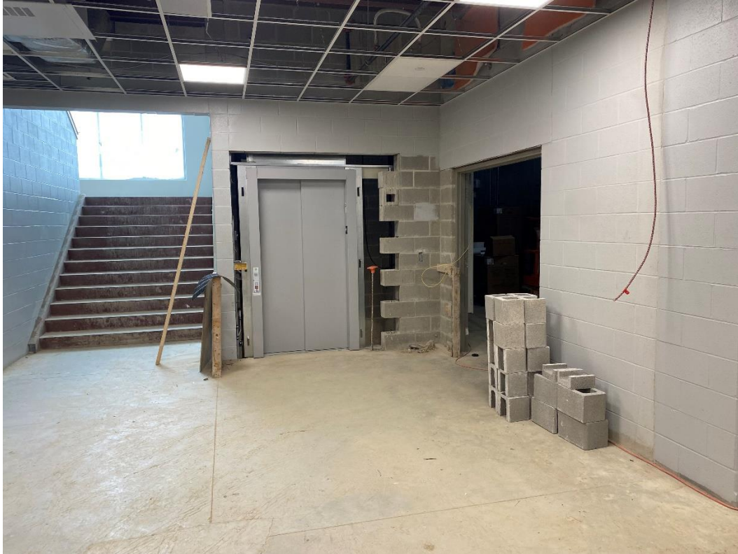
The elevator installation is complete. Masons will finish block work around the doors.
