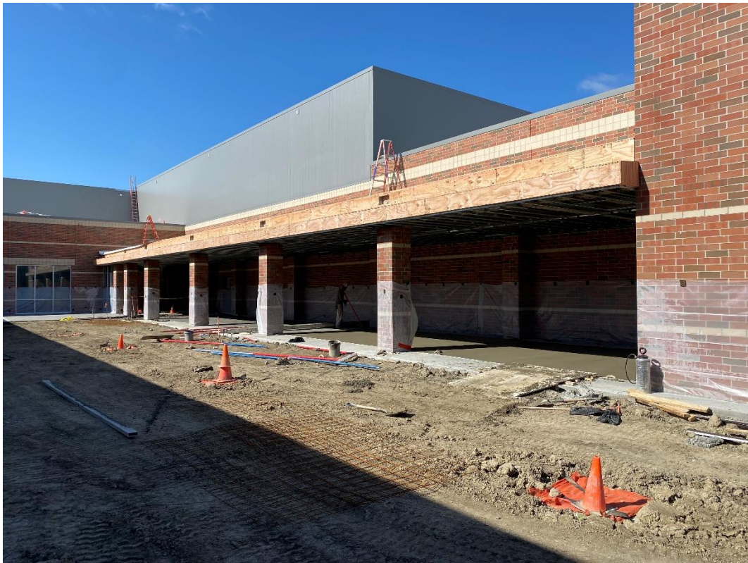
North entry slab/walk is installed. This will be the construction entry starting next week.
