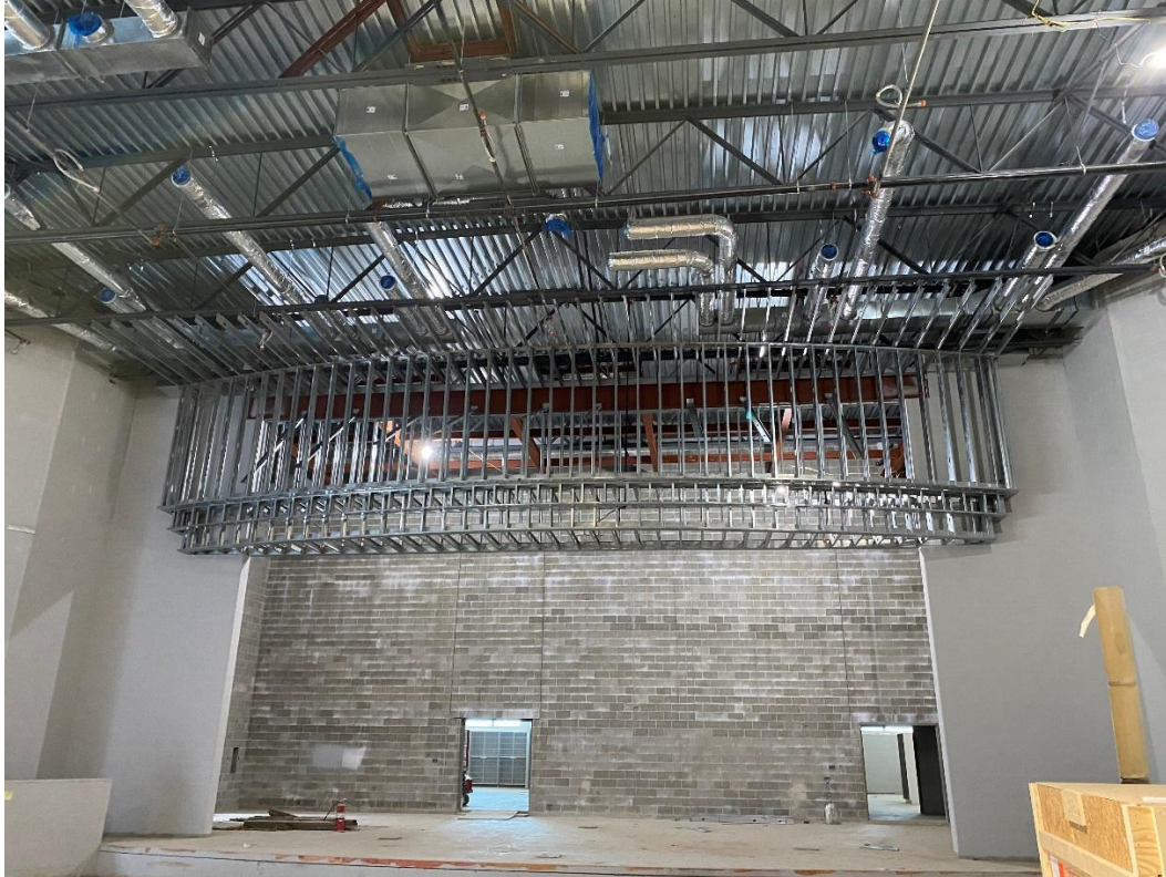
Framing of the curved face soffit above the stage is complete, drywall to follow.
