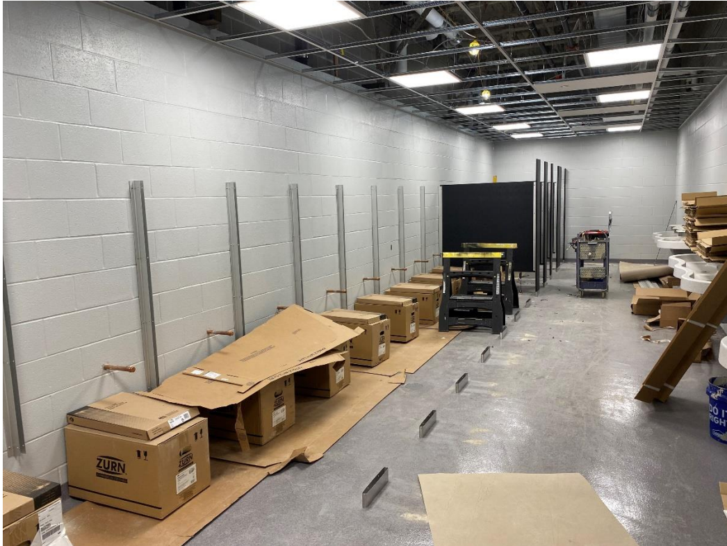
Installation of toilet partitions in the main toilet rooms will be complete this week.
