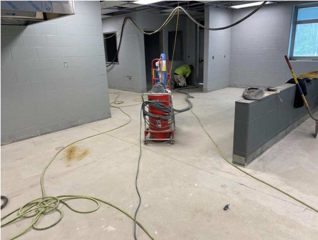
Kitchen floor slab is being ground in preparation for epoxy floor finish.
