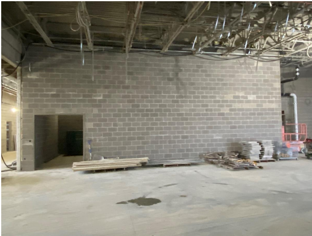
Masonry is complete at the Chair Storage room north of the Gym.
