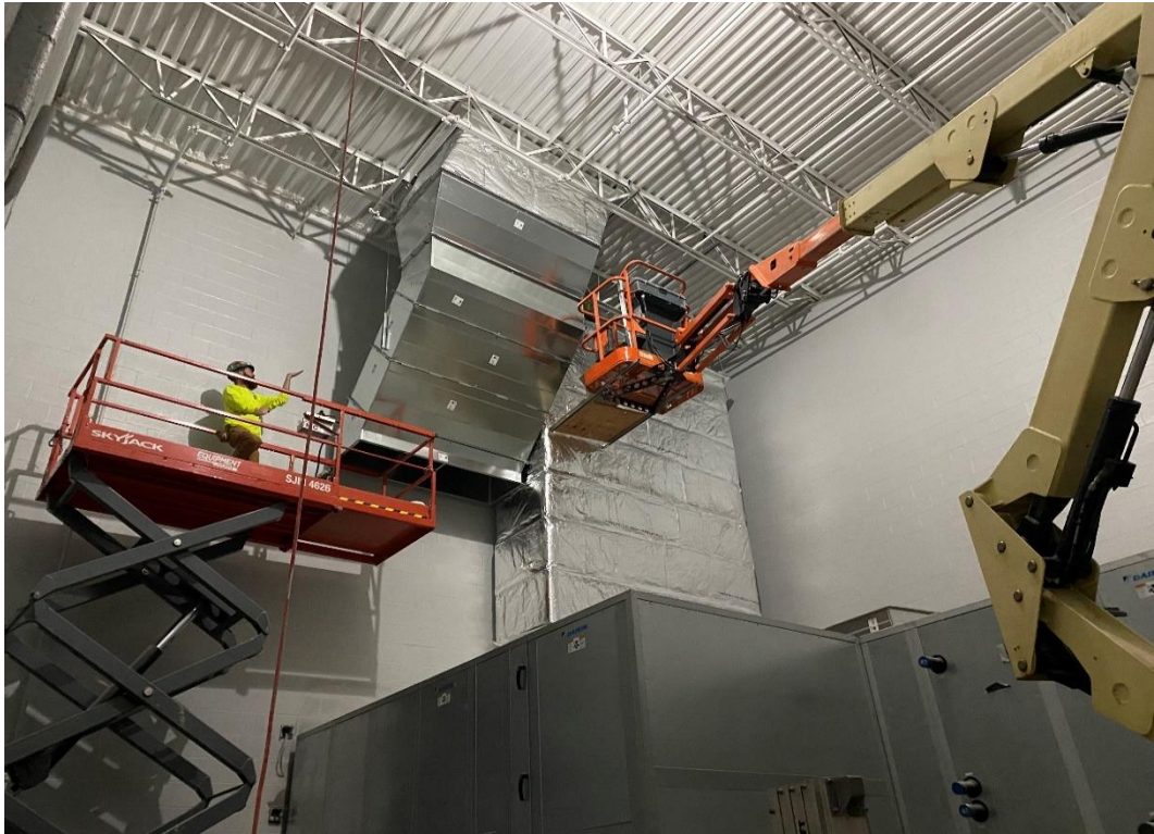
Fresh air ductwork and ductwork from the roof-top ventilator is being installed and insulated in the Area C Mechanical Room.
