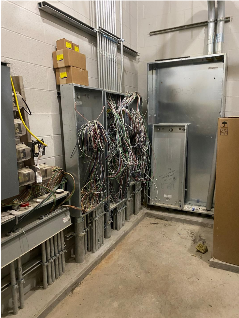
Panelboards and circuit wiring is being installed to the panels in the main electrical room at Area D.
