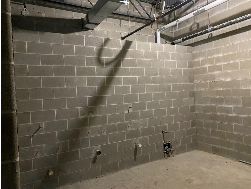
Interior masonry walls at the first-floor toilet rooms in Area C are complete.
