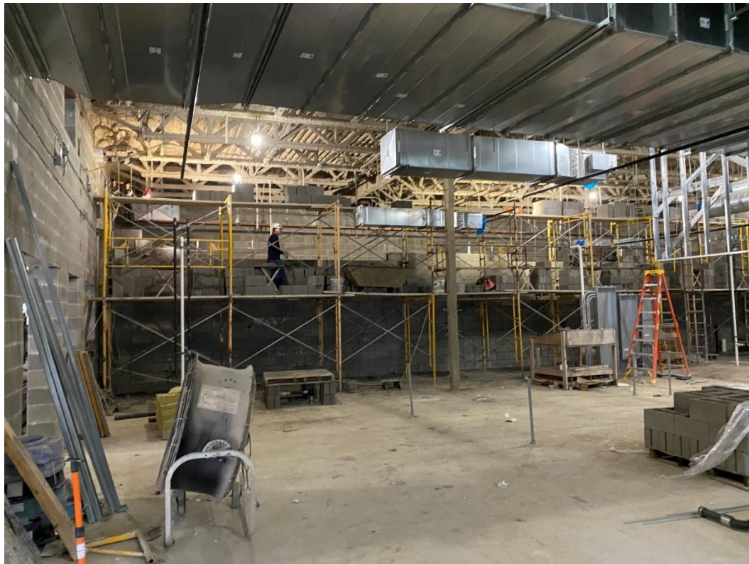
The masonry wall at the freezer/cooler in the Kitchen is nearly complete.
