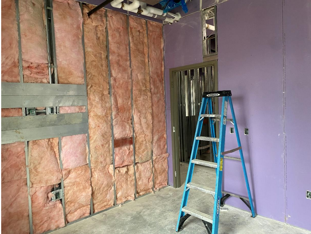
Installation of acoustical insulation and drywall has begun in the Administrative Offices.
