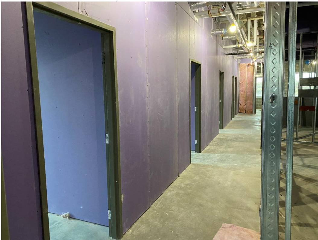
Drywall installation is progressing at the east offices in the Administrative Office area.
