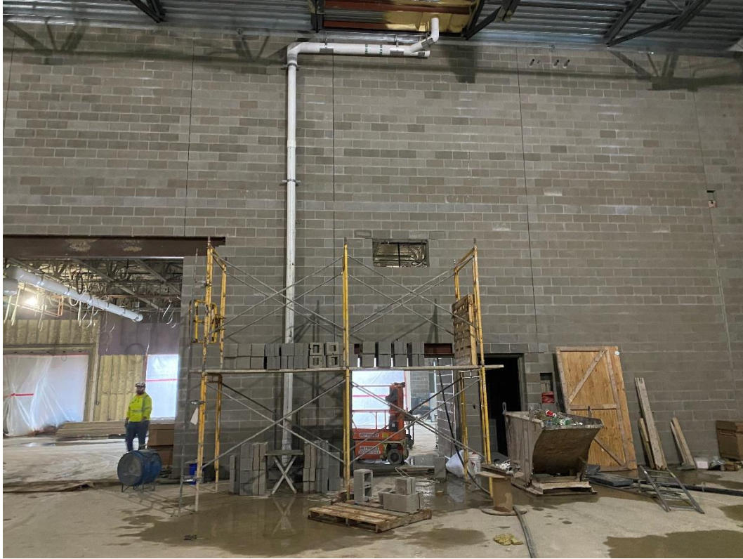
Masons have started the enclosure of storm drainage piping in the Gym. View looking north.
