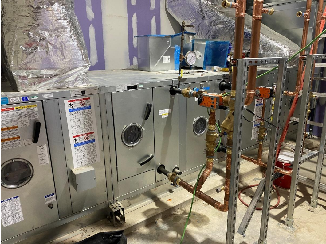
The air handling unit for the Administrative Offices is being plumbed with hydronic piping.
