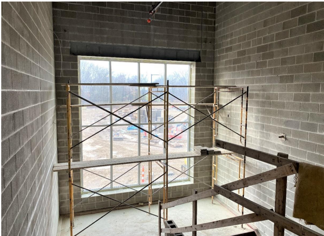
Scaffolding is being constructed for installation of masonry at the beam above the large window (to the west) at the main stair to the second-floor of Areas C & D.
