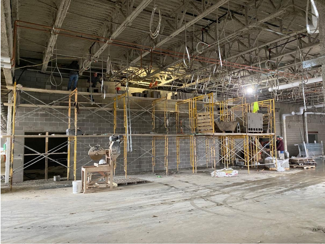
Masonry walls of the Chair Storage room are nearly complete to the underside of the structure above.
