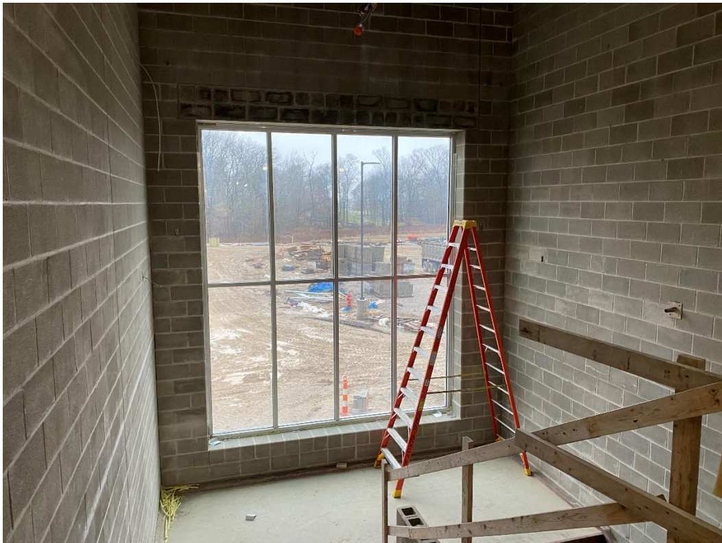
Masonry above the large window at the main stair in Area C is complete and scaffolding has been removed.
