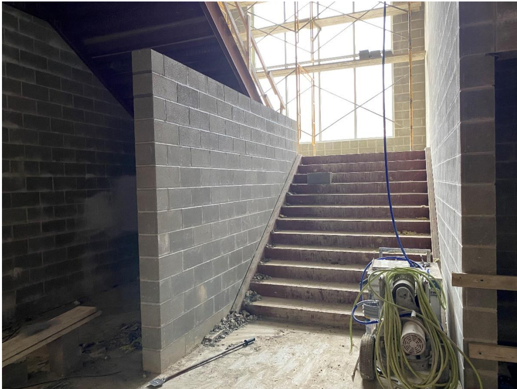
Construction of the stair railing wall is progressing at the main stair at Area C.
