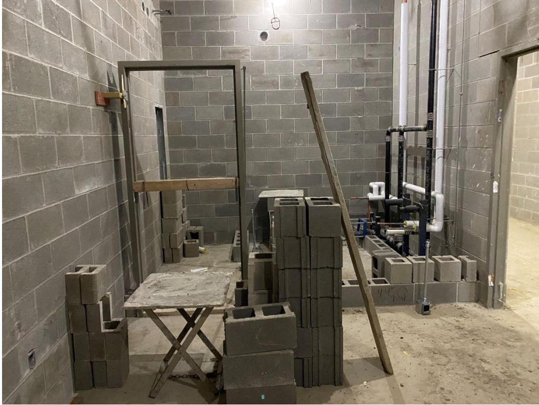
View looking west toward the Staff Shower in the Area E, Locker Rooms. Plumbing Rough-in is complete and insulated.
