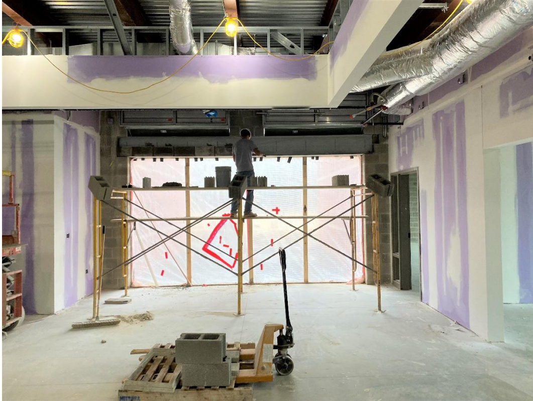
Concrete masonry is being installed at the large beam at the north first-floor exit from Classroom Area D.
