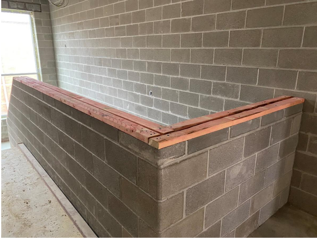
Fire treated wood blocking is installed at the stair railing wall of both (minor) stairs at Areas C & D.
