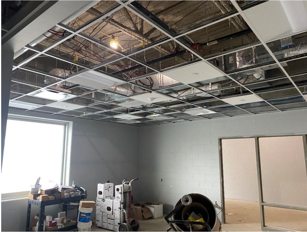
Ceiling grid, lighting, HVAC diffusers, sprinkler heads and alarms is complete in Area A.
