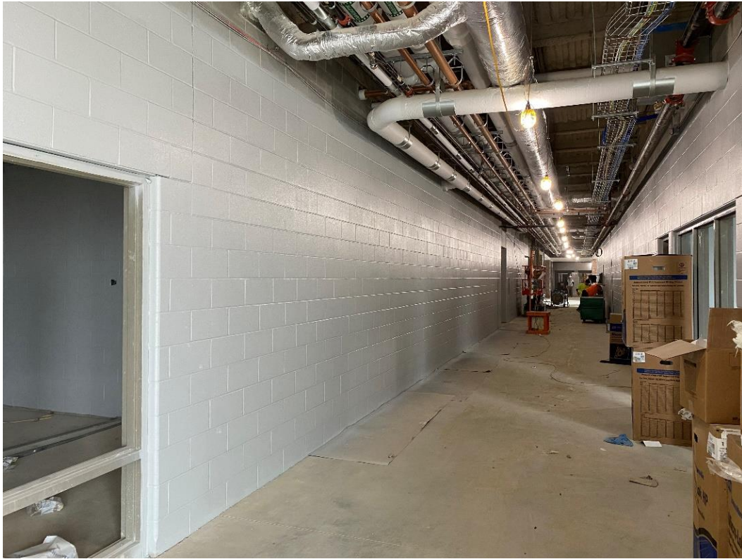
Corridor walls are painting in the main corridor east of the Gym.
