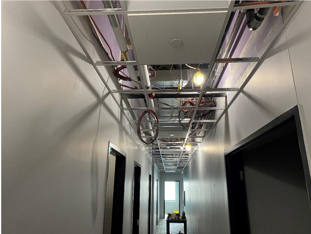
Ceiling grid, lighting, HVSAAC diffusers and sprinkler heads are installed in Area A corridors.
