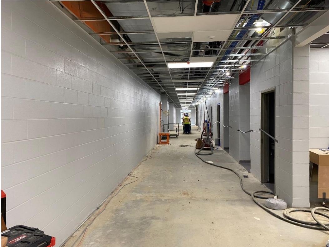
First floor ceiling grid is installed in Area C & D main corridor.
