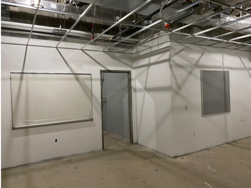
Ceiling grid, marker and tack boards are installed in the :Locker Rooms.
