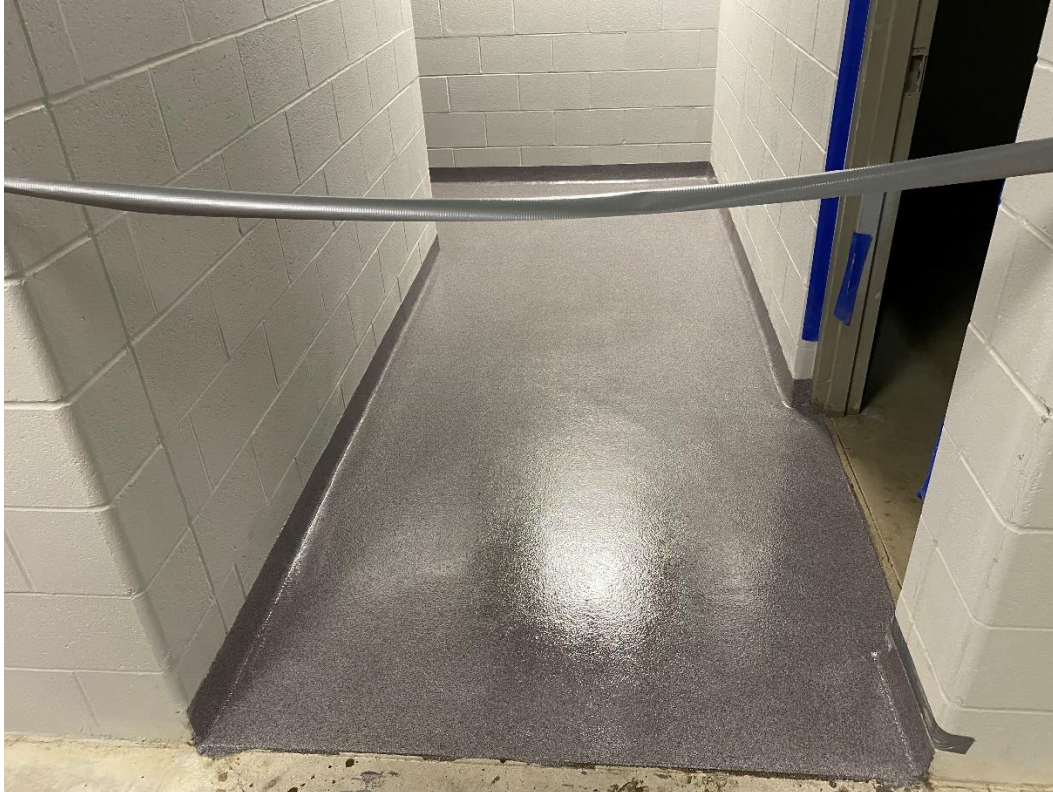
Epoxy floors are completed in the main toilet rooms, Area C, first-floor.
