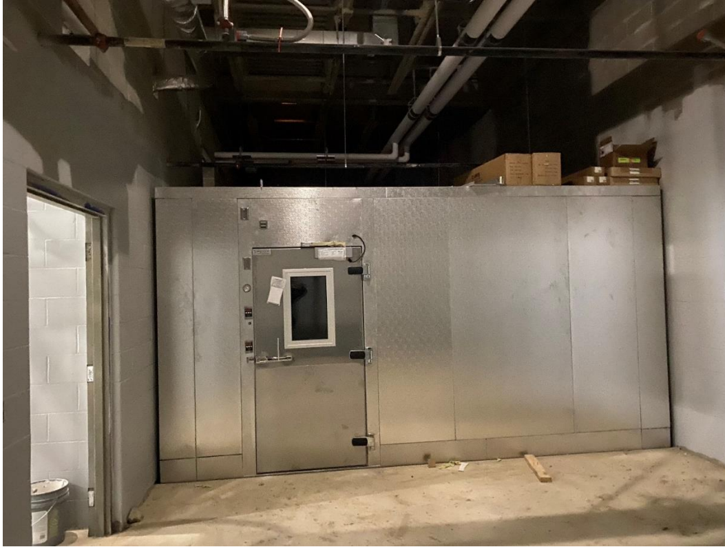
The freezer/cooler for the Kitchen is assembled. Floor slab to be installed next week.
