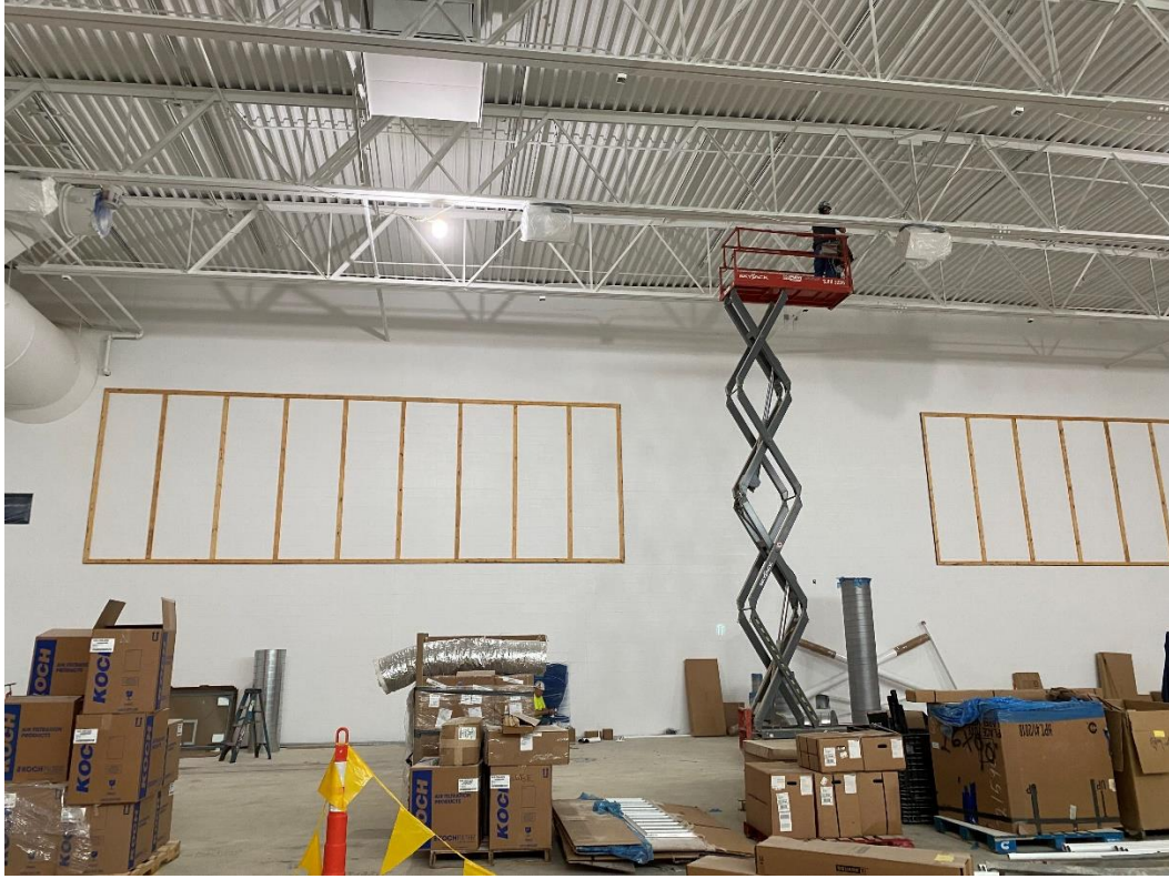
Speakers are wired and blocking for acoustical panels is installed on Gym walls.
