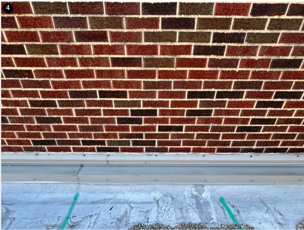
Section C - 2 wet areas are present along the wall. The through wall flashing is questionable along the wall.
