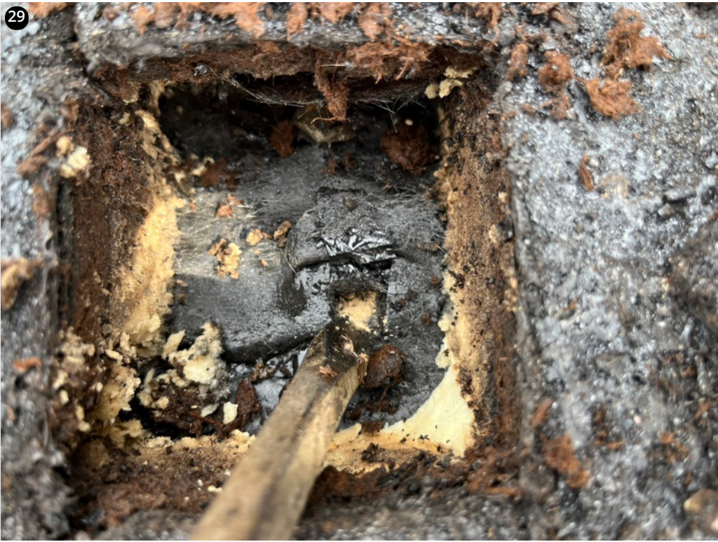
Section D, Core Cut = flat tectum deck + ISO + CB + BUR and gravel.
