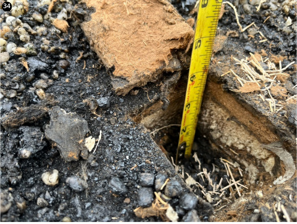
Section E, Core Cut = flat tectum deck + CTP and Gravel + insulation + BUR and gravel .
