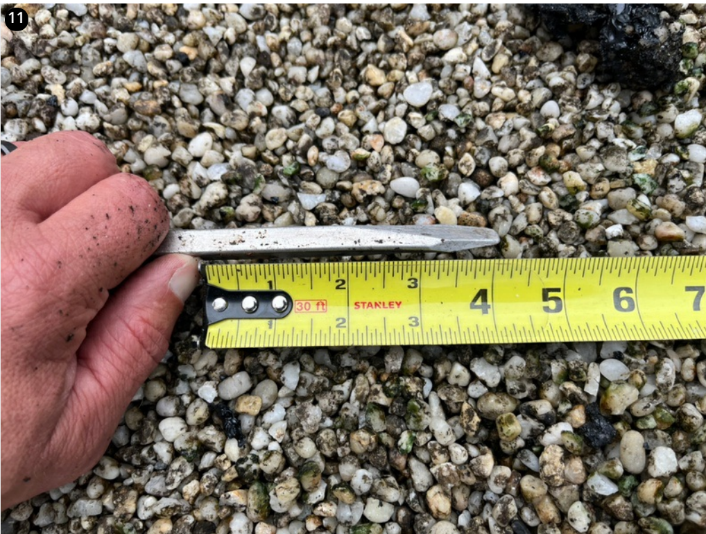
11 The depth of the roof near the drain is 4 inches. Tapered insulation is needed.
