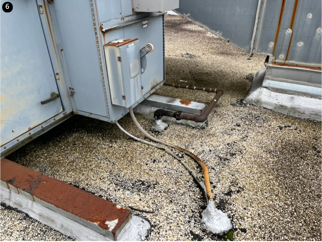
The gas pipe likely needs to be raised.
