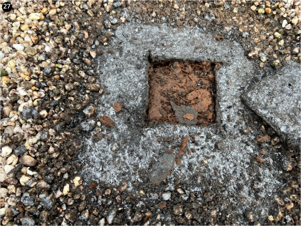
Section D - the core cut revealed wet insulation.
