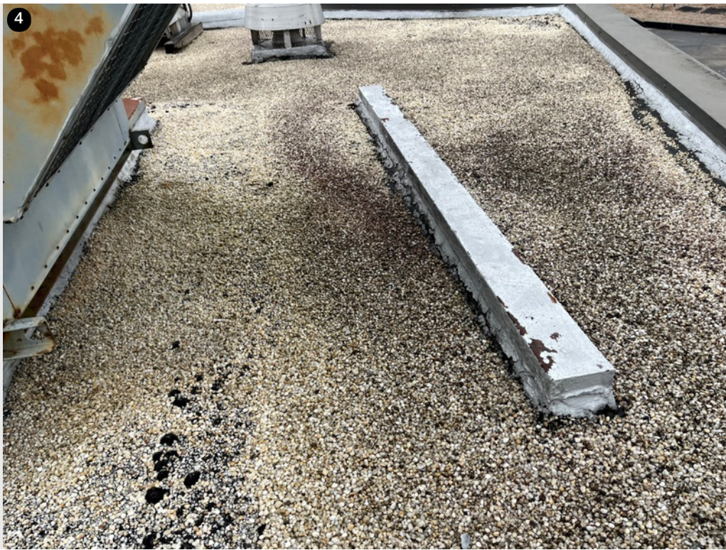
The obsolete curb needs to be removed.
