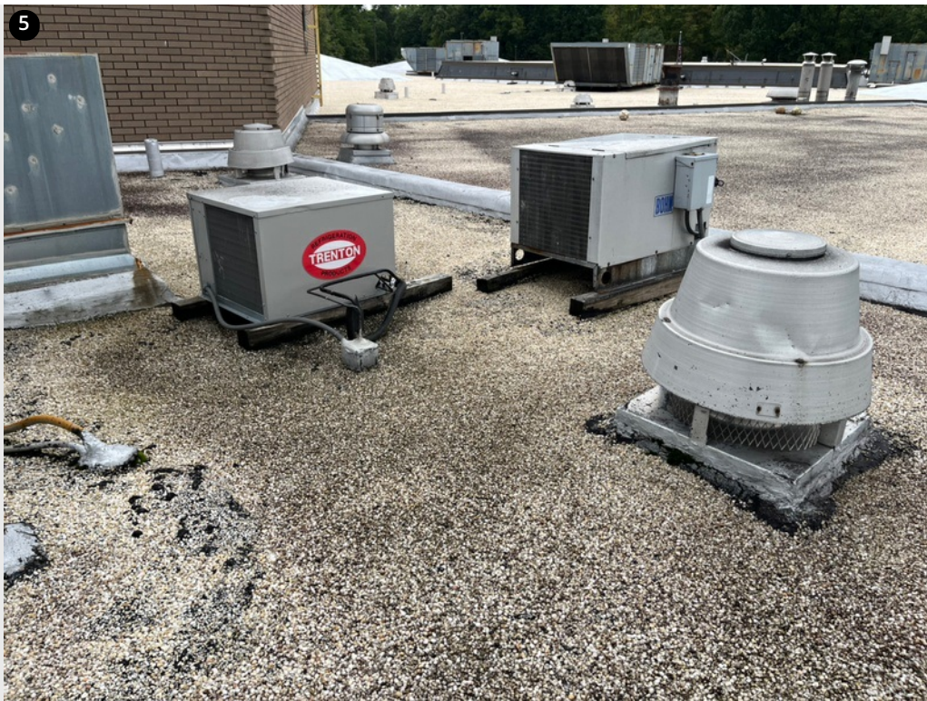
The fan units need to be raised.
