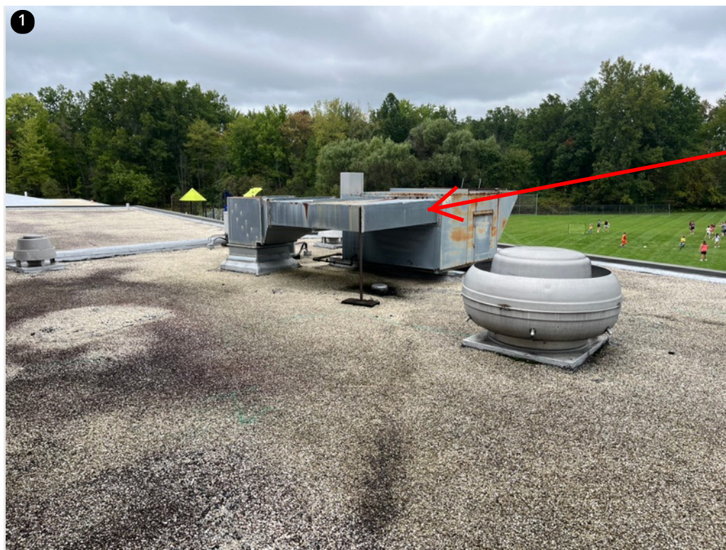
Overall roof photo. The unit and fans need to be raised.
