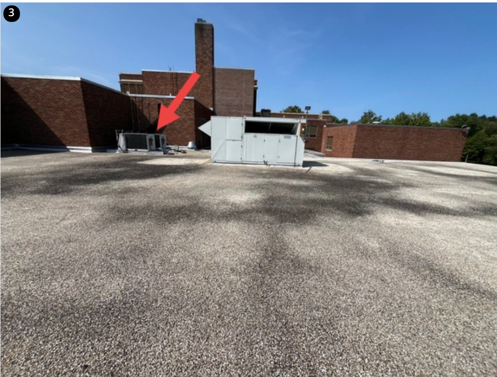
Section C - overall roof photo. The units on the left need to be raised. The roof is difficult to access under the units and the roof height will be raised with the new tapered insulation.
