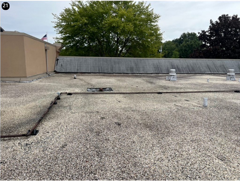
Section D - overall roof photo. Per the roof scan and limited core cuts the wet areas are located on this roof section.
