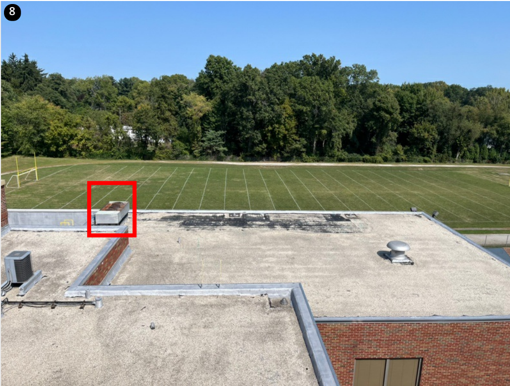
Section F - overall roof photo. The unit may need to be raised to accommodate the new tapered insulation height.
