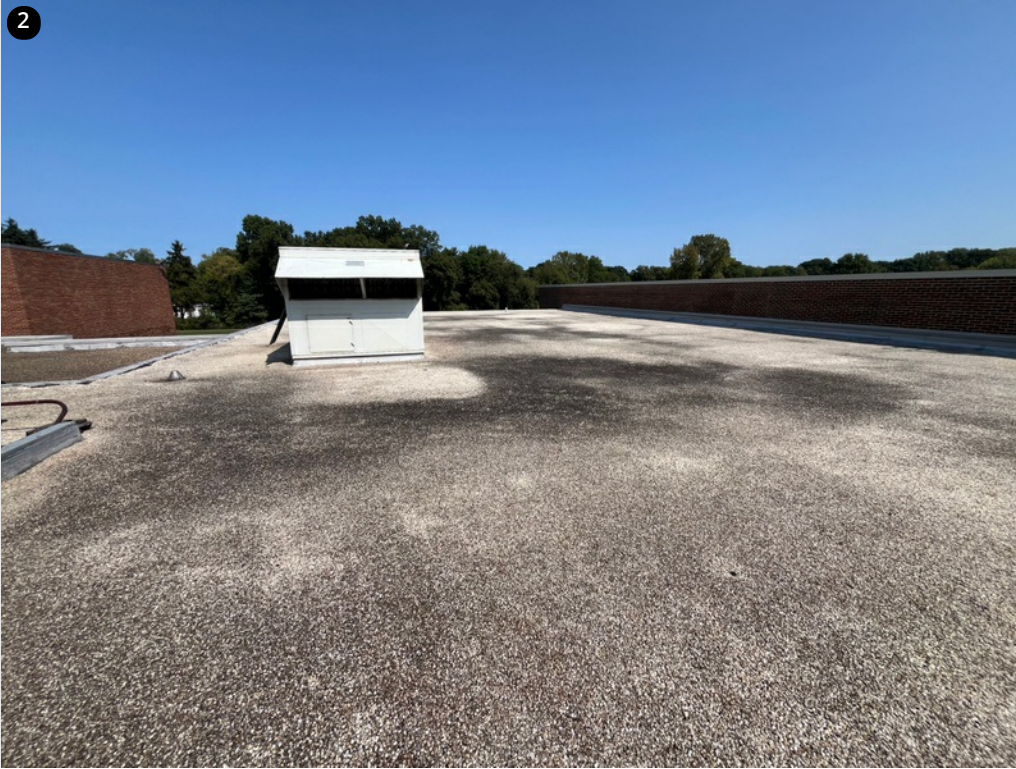
Section C - overall roof photo. Flashing height is limited around the large HVAC unit.
