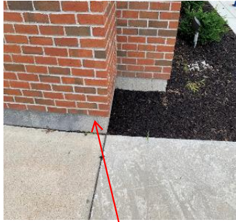
Crack at foundation.
