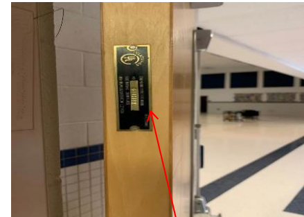
Typical rated corridor door.
