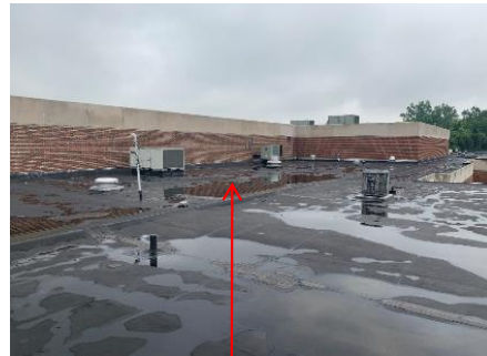
Areas of ponding.
