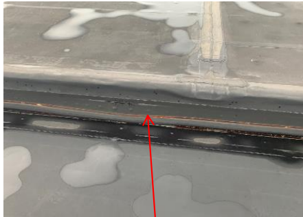
Rusting roof flashing and joint opening up.
