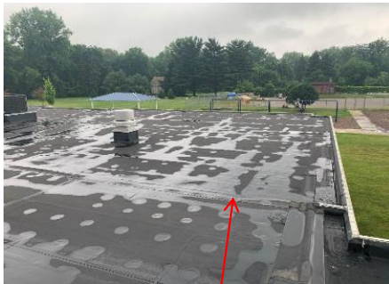
Areas of ponding.
