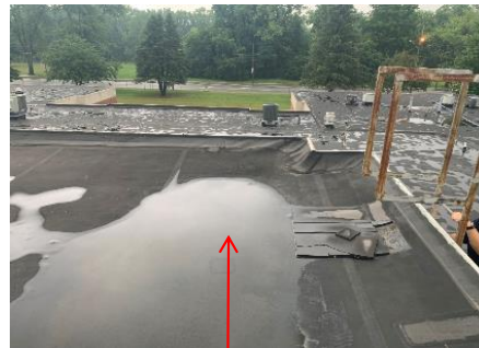
Areas of ponding.
