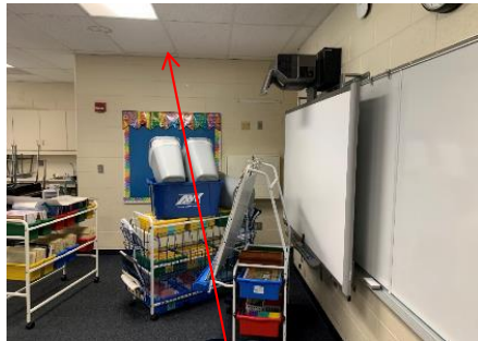
Stained ceiling tiles.
