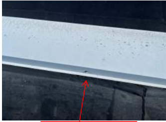
Loose metal coping fastener.
