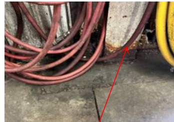
Rusting Steel Bldg Frame
