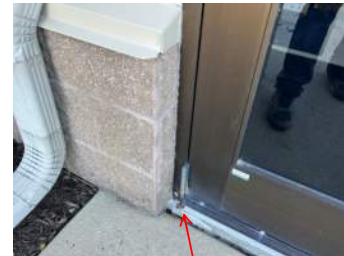
Damaged door threshold / door frame corrosion
