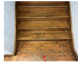
Flooring in Poor Condition
