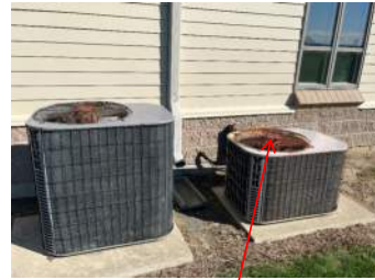
Rusting HVAC equipment
