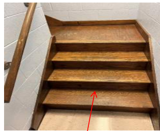
Flooring in Poor Condition
