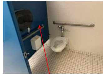
Missing vertical grab bar.
