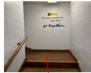
Flooring In Poor Condition
