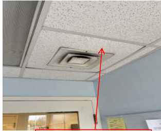
Rusting HVAC Diffuser
