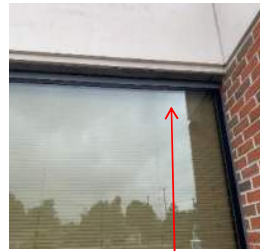
Open joint at window head.
