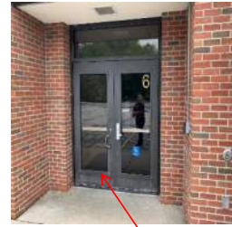
Damaged entry doors.
