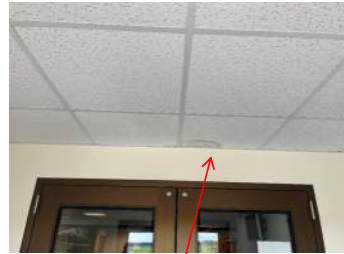
Damaged ceiling tile
