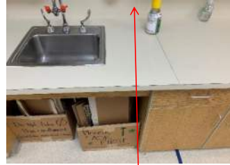
Damage to plastic laminate countertop.
