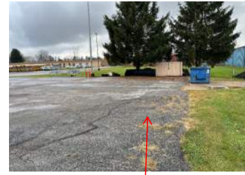
Poor Asphalt Condition
