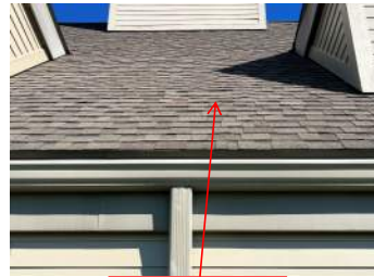
Roof shingle damage
