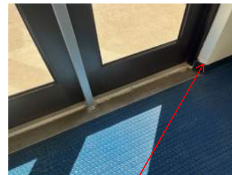
Damaged gyp. board wall and loose wall base.
