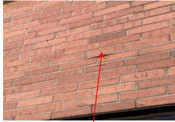
Damaged masonry and mortar joints.
