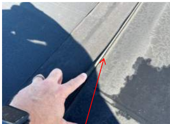
Loose roofing joint/seam.
