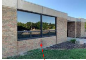
Staining on masonry.
