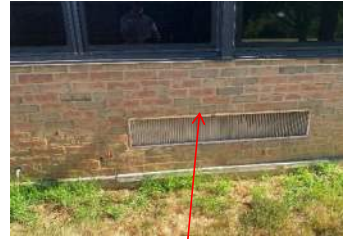
Repair / replace louver and re-seal.
