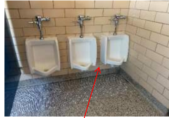
Urinal installation is not ADA compliant.
