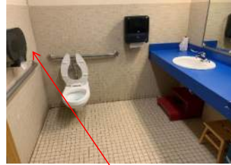
Missing vertical grab bar.
