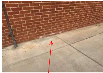
Damage at masonry.
