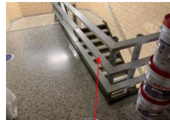
Stair railing is not Building Code compliant.
