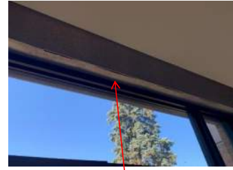
Damage at window head.
