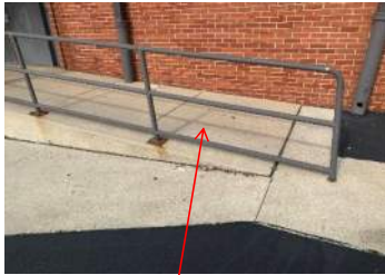
Rusting at handrail / anchor plates.
