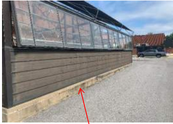
Damage at foundation - replace concrete coating.
