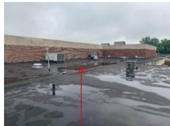
Areas of ponding.
