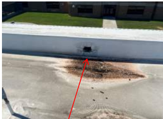
Signs of ponding water and roof overflow may set too high.
