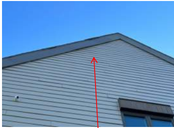
Damaged metal eave wrap
