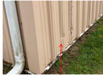
Damaged Metal Siding
