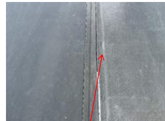
Roofing joint/seam cracking needing repair.
