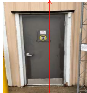
Damaged Door Head
