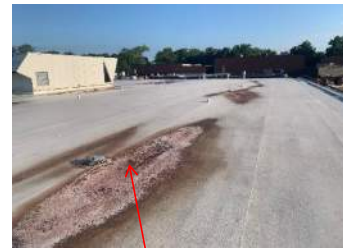
Ponding on roof.
