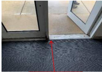
Damage at door frame.
