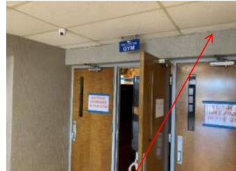
Damaged ceiling tiles.
