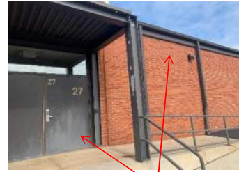
Damage at entry door. Chipped/peeling paint at entry canopy frame.
