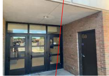
Joint opening up.
