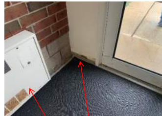
Damage to flooring base. Rusting HVAC unit.
