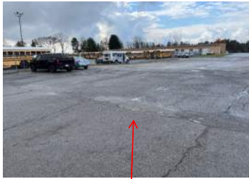
Poor Asphalt Condition
