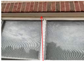
Rusting at lintel.
