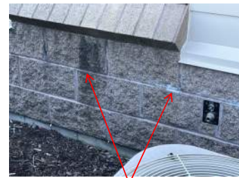
Masonry staining and efflorescence
