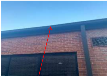
Damage at gutter.
