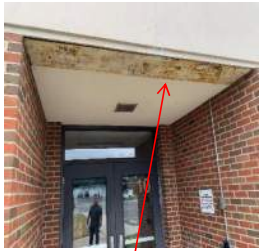
Rusting lintel at entry.
