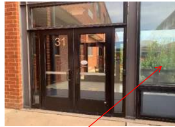
Seal broken on insulated glazing.
