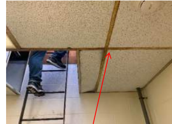
Rusting ceiling grid.
