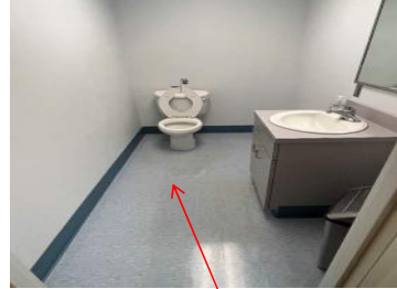
Restroom not ADA compliant
