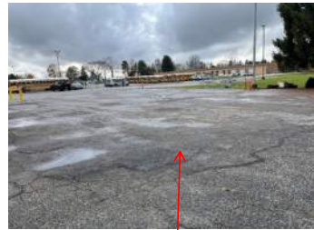
Poor Asphalt Condition
