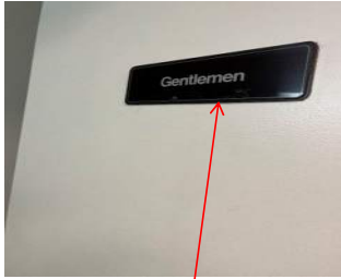
Signage Not Compliant
