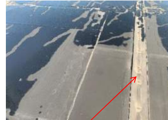
Damaged roofing material - several repairs due to wind.
