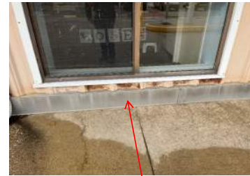
Rusting Metal Siding
