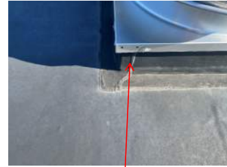
Roofing joint/seam cracking needing repair.
