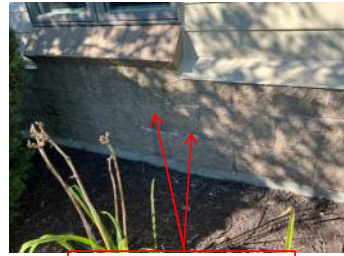
Masonry staining and efflorescence
