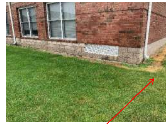
Missing downspout splash block.
