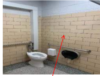
Missing vertical grab bars.
