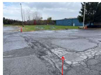
Poor Asphalt Condition
