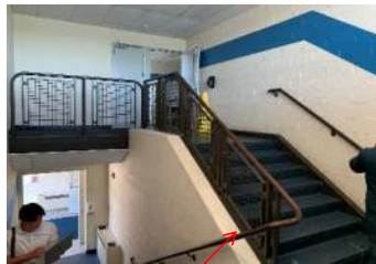
Stair railing is not Building Code compliant.
