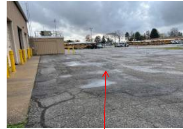
Poor Asphalt Condition
