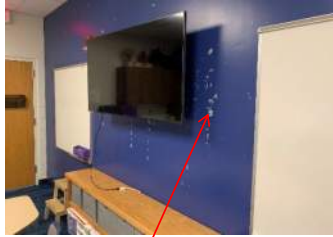
Repair / repaint walls.
