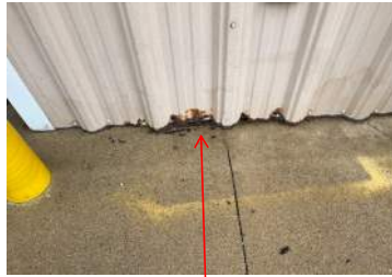
Rusting Metal Siding
