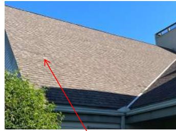
Roof shingle damage
