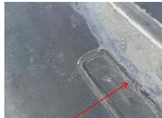
Roofing joint/seam cracking needing repair.
