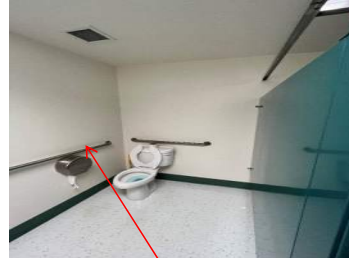
Missing vertical grab bar
