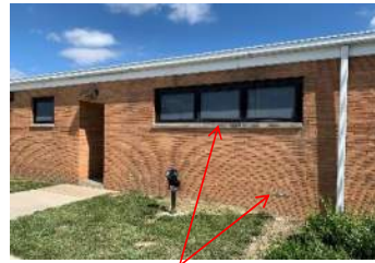
Masonry repairs and staining.
