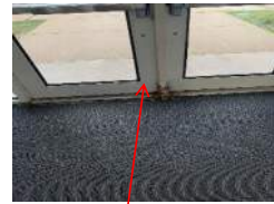
Damage to door frame.
