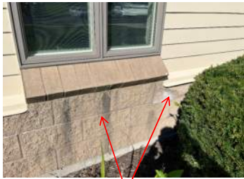
Masonry staining and efflorescence
