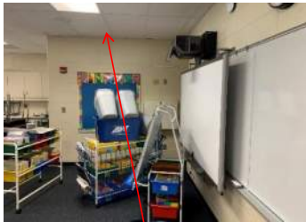
Stained ceiling tiles.
