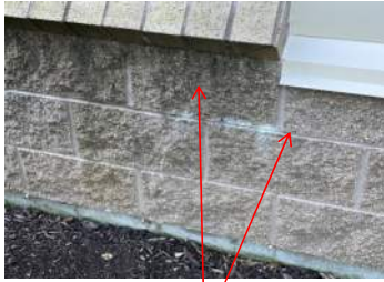
Masonry staining and efflorescence
