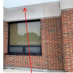
Staining on exterior wall.
