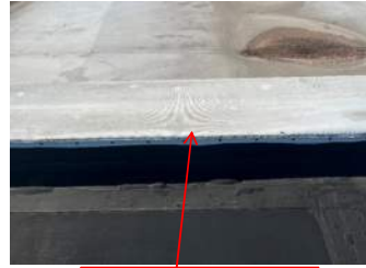
Term bar sealant needs replaced.
