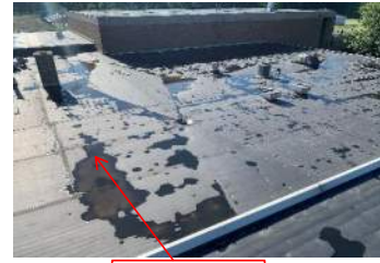
Ponding on roof.
