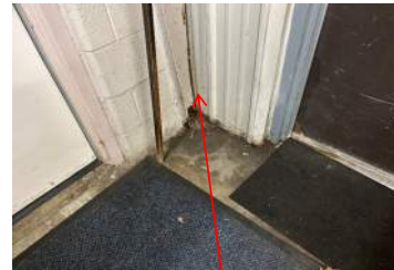
Rusting Steel Bldg Frame
