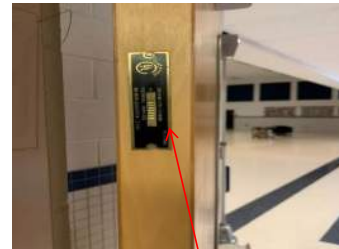
Typical rated corridor door.
