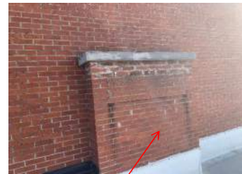
Masonry repairs and staining.
