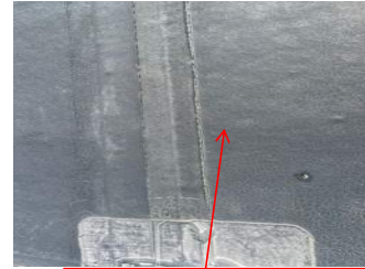
Roofing joint/seam cracking needing repair.
