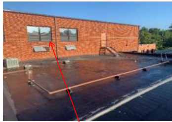
Rusting at vent.
