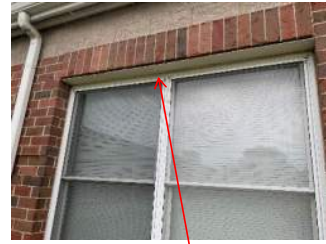
Rusting at lintel.
