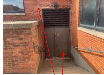
Masonry repairs. Rusted entry door.
