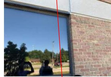
Need repairs at window head.
