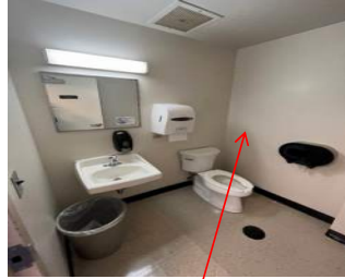
Missing Grab Bars
