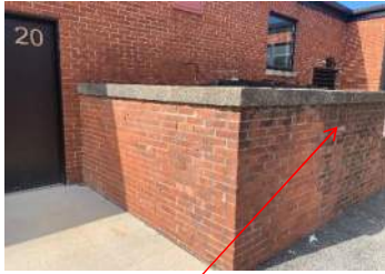
Masonry repairs and staining.
