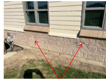
Masonry staining and efflorescence
