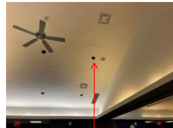
Damaged / crack in gyp. board
