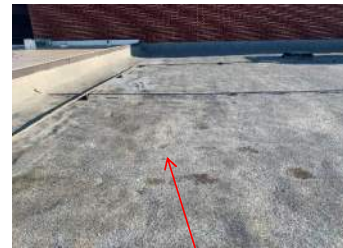
Older section roof - nearing end of life.
