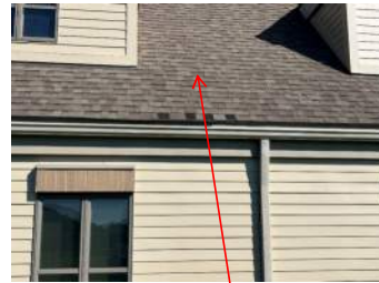
Roof shingle damage
