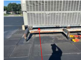
Rusting roof equipment.
