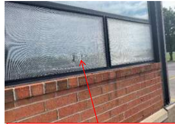
Staining at window sill and damaged window screen.
