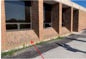
Staining on masonry.
