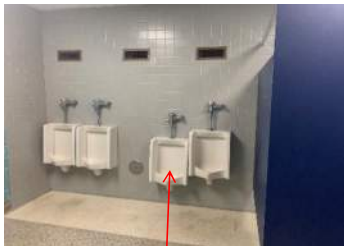
Urinal installation is not Building Code compliant.
