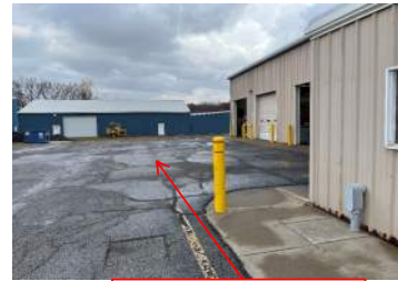
Poor Asphalt Condition
