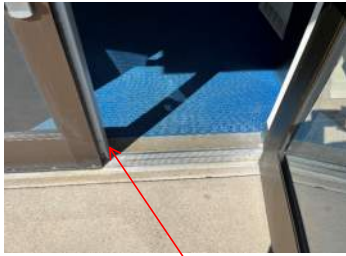
Damaged door threshold / door frame corrosion / rusting door mullion
