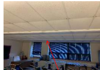
Sagging ceiling tiles.
