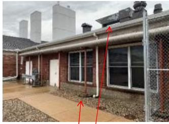
Peeling paint on mechanical units. Rusting at columns and bases.
