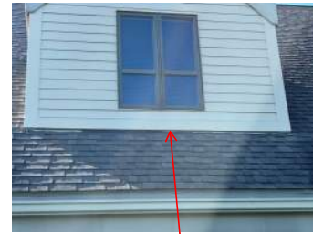
Roof flashing in poor condition
