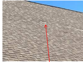
Roof shingle damage
