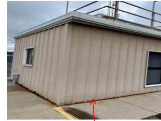
Rusting Metal Panel
