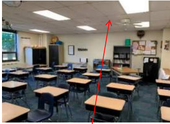
Sagging ceiling tiles.
