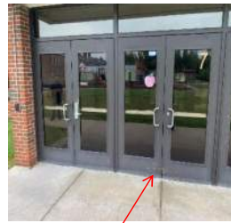
Damaged entry doors.
