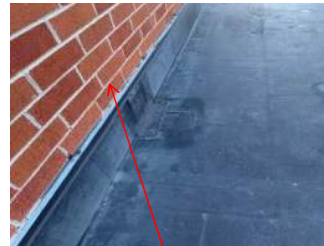
Failing sealant joint at flashing
