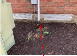
Missing downspout splash block.
