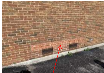
Damaged masonry and mortar joints.
