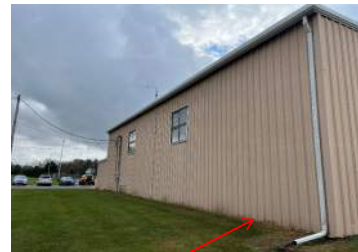
Rusting Metal Panels
