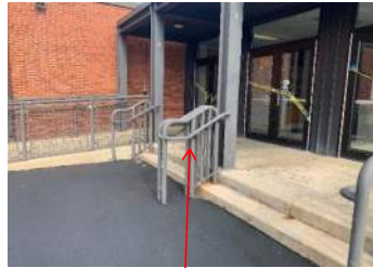
Rusting at handrail.
