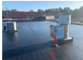
Rusting at rooftop equipment.
