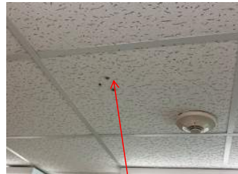
Damaged ceiling tile
