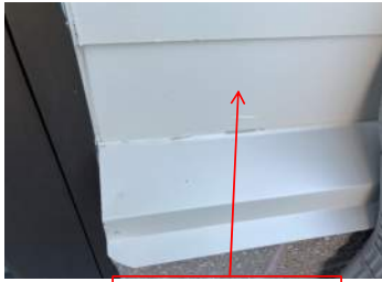
Open joint in wall cap flashing
