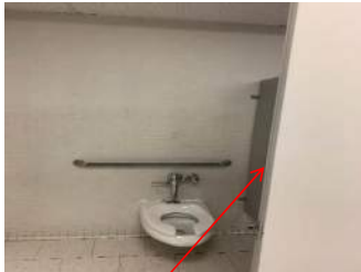
Missing grab bars.
