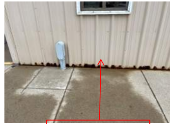
Rusting Metal Siding
