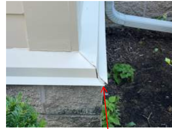
Open joint in wall cap flashing
