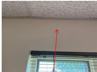
Damaged / crack in gyp. board
