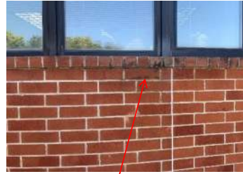
Staining at window sill.
