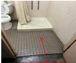
Flooring in Poor Condition
