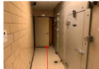
Rusting at bottom of door.
