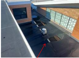
Ponding water present.
