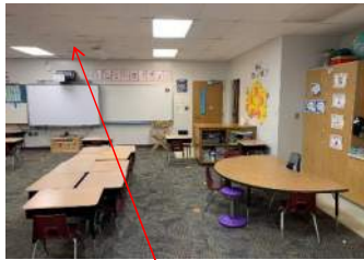
Sagging ceiling tiles.
