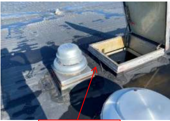
Rusting at roof vent.
