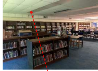
Damaged ceiling tiles.
