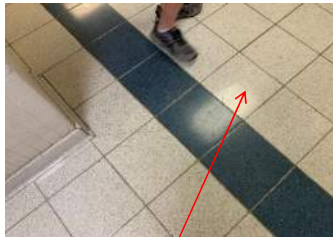
Cracks in flooring.
