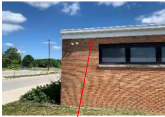
Damaged masonry and mortar joints.
