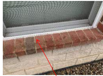
Failing sealant joint at window sill.
