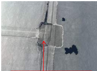
Roofing joint/seam cracking needing repair.
