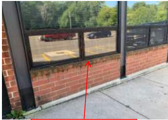
Masonry repairs and staining.
