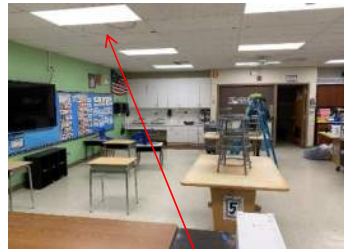
Stained ceiling tiles.
