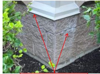
Masonry staining and efflorescence
