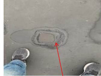
Failing roof patch joints/cement.
