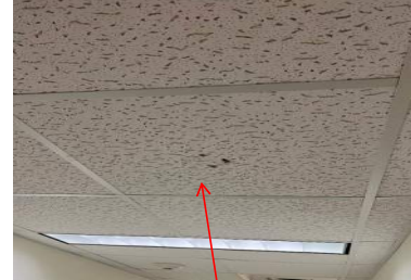
Damaged ceiling tile
