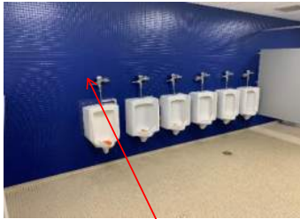
Need to repair tile at urinals.
