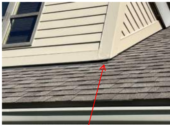
Damaged roof flashing & damaged siding materials
