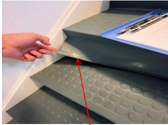
Loose stair finishes
