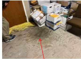
Water stains from roof leak in attic
