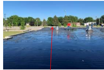
Ponding on roof.
