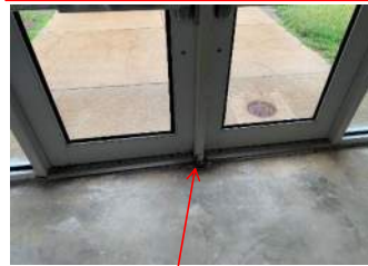
Damage to door frame.
