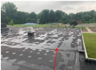
Areas of ponding.
