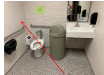
Missing vertical grab bar.
