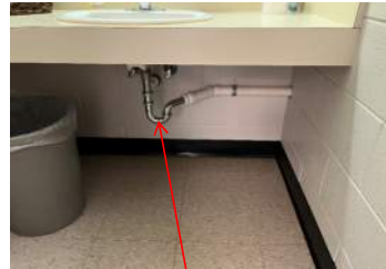
Need Piping Protection
