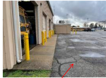
Poor Asphalt Condition
