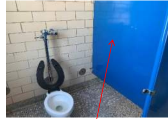
Missing grab bars.
