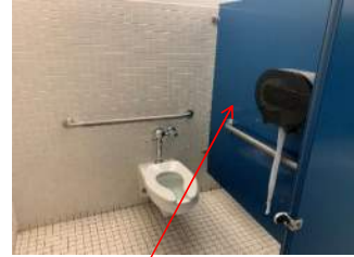
Missing vertical grab bar.
