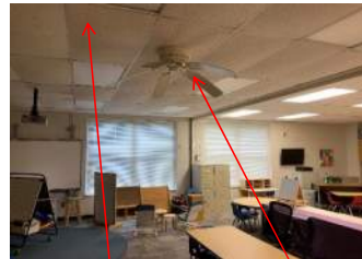
Sagging ceiling tiles
