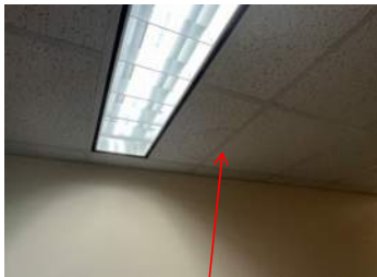
Damaged ceiling tile
