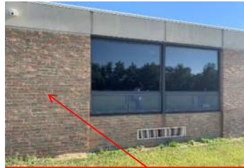
Rough brick at middle section of wall. Cracking and popping.
