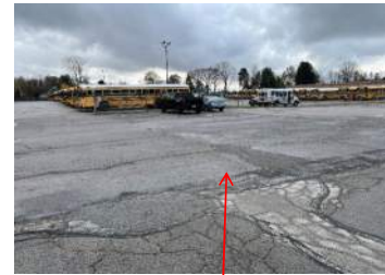
Poor Asphalt Condition
