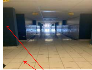
Cracks in flooring and carpet on corridor walls.
