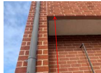
Damage at soffit.
