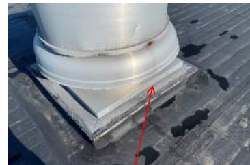
Damaged roof vent. Need to repair caulk joint.
