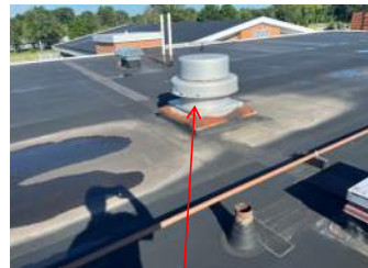
Rusting roof equipment.
