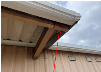
Rusting Steel Framing
