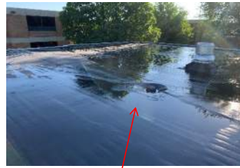
Ponding on roof.
