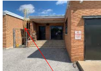
Repaint roof access ladder
