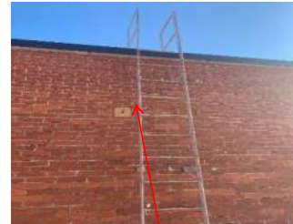
Loose anchor on ladder and needs painted.
