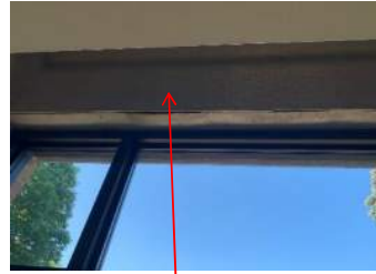
Damage at window head.
