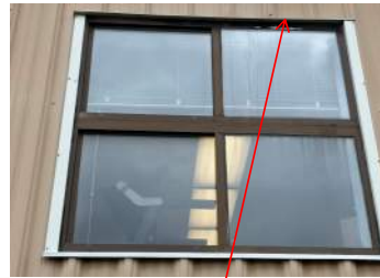
Window Finish Failing
