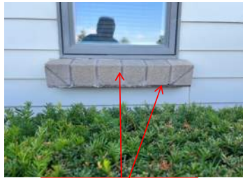
Rusting lintel and efflorescence
