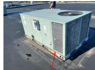
Rusting roof equipment.
