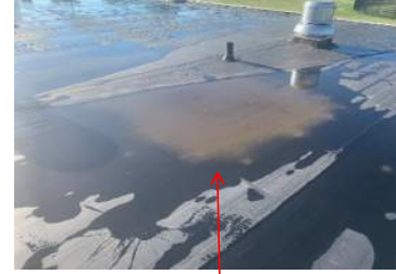
Areas of ponding.
