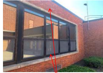
Staining on window sill - masonry repair tuck point.
