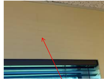
Damaged / crack in gyp. board
