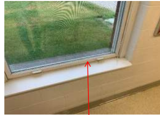
Extremely large operable windows making opening and shutting very difficult
