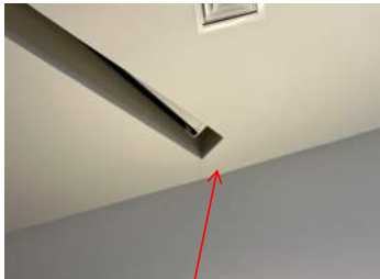
Damaged / crack in gyp. board
