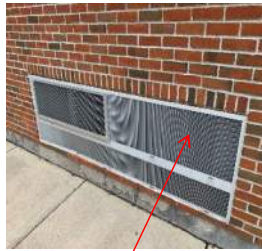
Caulk joint at top of louver.
