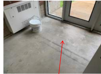
Missing walk-off carpeting at doors.
