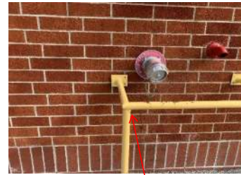
Missing anchors and rusting at guard.
