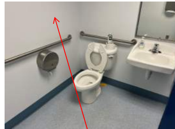
Missing vertical grab bar
