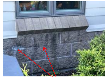
Masonry staining and efflorescence
