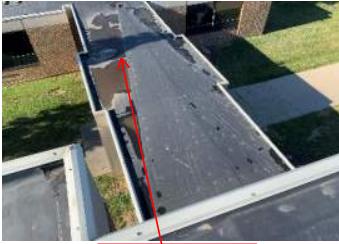
Ponding on roof.
