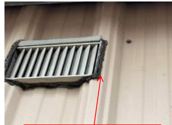
Failing Sealant - Replace Louver
