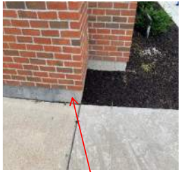
Crack at foundation.
