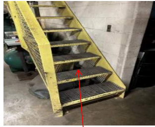
Stair Not Complaint
