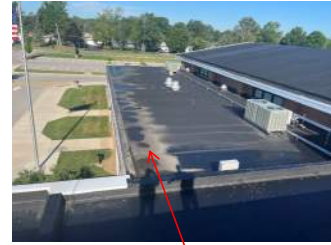
Ponding water present.
