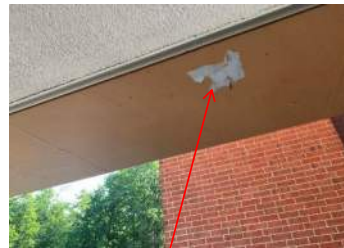
Peeling paint at soffit.
