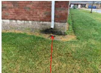
Missing downspout splash block. Staining at wall.
