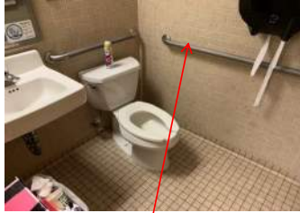
Missing vertical grab bar.
