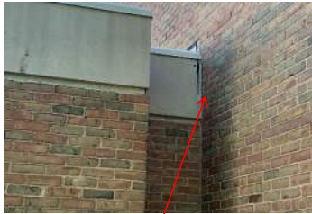
Open joint - re-seal.
