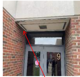
Peeling paint at entry.
