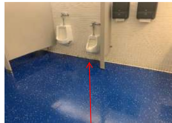
Damaged ceramic tile wall base.
