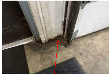
Rusting Interior Metal Panel
