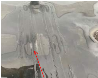
Failing roof patch joints/cement.
