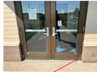
Damaged door threshold / door frame corrosion
