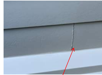
Open joint in siding
