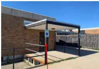
Chipping/peeling paint at entry canopy.
