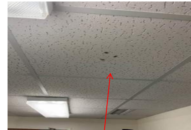
Damaged ceiling tile
