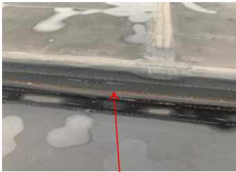
Rusting roof flashing and joint opening up.
