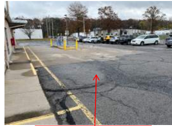
Poor Asphalt Condition
