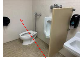
Missing grab bars.
