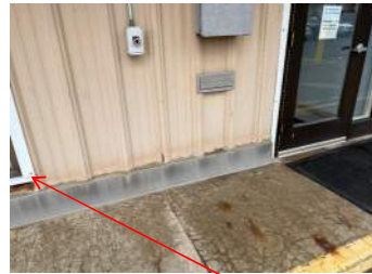
Rusting Metal Siding
