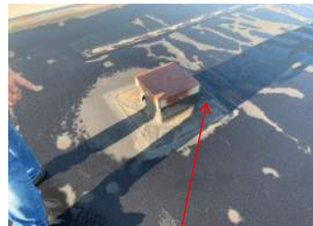
Rusting at penetration/cap.
