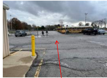
Poor Asphalt Condition
