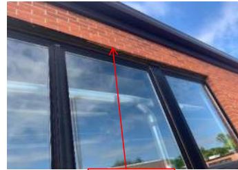
Rust at lintel.
