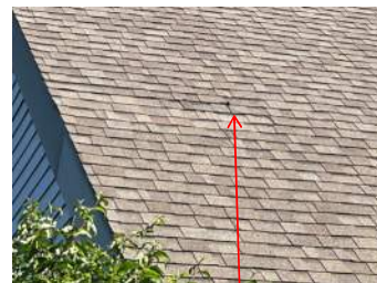
Roof shingle damage
