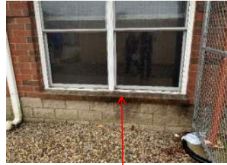
Staining at window sill.
