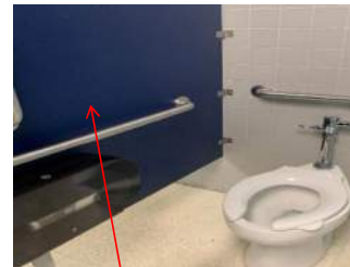
Missing vertical grab bar.
