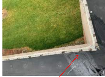
Failing roof cement/joints.
