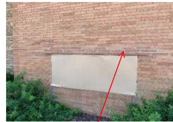
Need repairs at metal panel and masonry.
