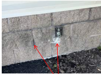
Masonry staining and efflorescence
