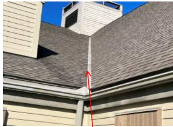
Roof flashing in poor condition
