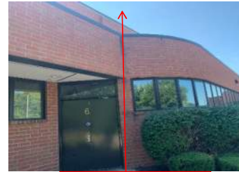
Masonry repairs and staining.
