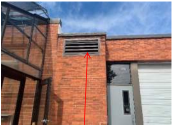
Masonry repairs and staining.
