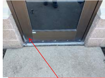
Damaged door threshold / door frame corrosion
