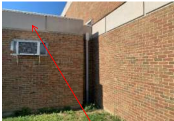
Rusted wall materials.
