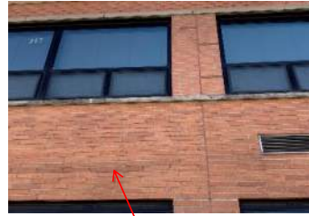
Damaged masonry and mortar joints.
