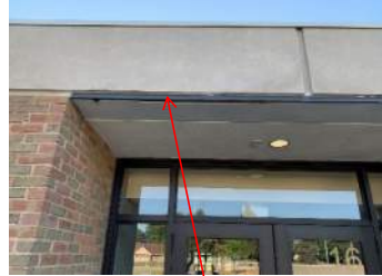
Joint opening up.
