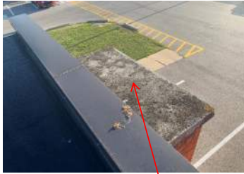
Staining on construction
