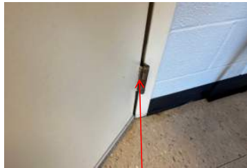
Rusting Door Hardware
