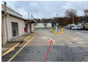
Poor Concrete Paving Condition
