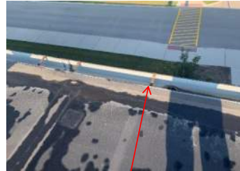
Rusting gutter anchors
