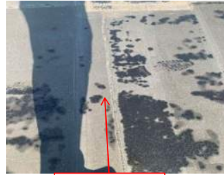
Failing roofing joint.
