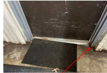
Rusting Interior Metal panels and door frame
