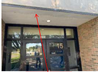
Joint opening up.
