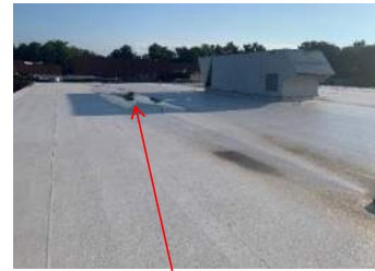
Ponding on roof.
