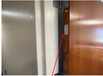
Typical rated corridor door
