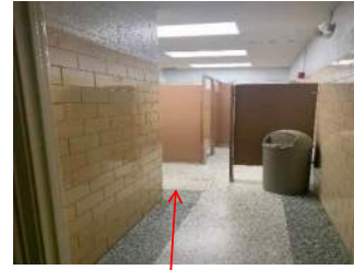
Corridor door has been removed, sight line and Building Code concerns.
