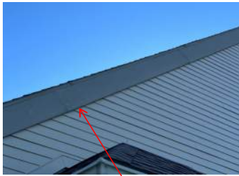
Damaged metal eave wrap
