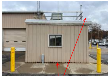
Rusting Metal Siding - Paint Roof Guard
