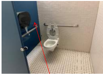
Missing vertical grab bar.
