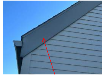
Damaged metal eave wrap
