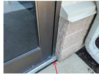
Damaged door threshold / door frame corrosion
