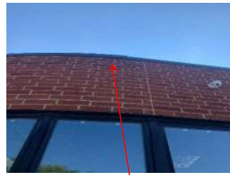
Damaged roof coping.
