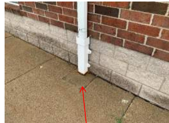
Rusting at downspout.
