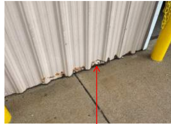
Rusting Metal Siding
