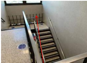
Stair railing is not Building Code compliant.
