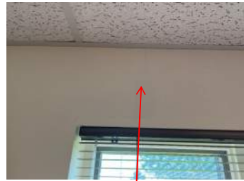
Damaged / crack in gyp. board
