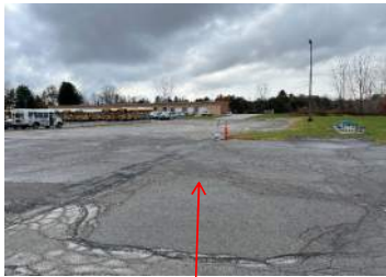
Poor Asphalt Condition
