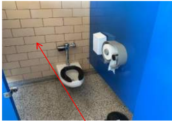
Missing grab bars.
