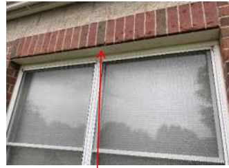
Rusting at lintel.
