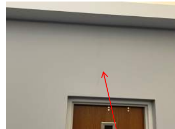
Damaged / crack in gyp. board
