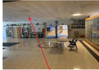
Sagging ceiling tiles.
