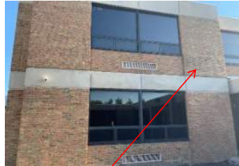
Staining on masonry.
