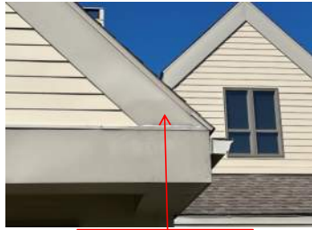
Existing metal trim repair
