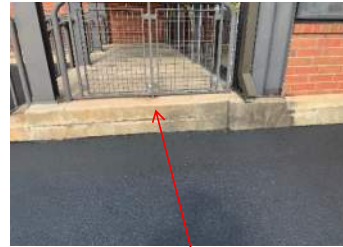
Damage at foundation - replace concrete coating.
