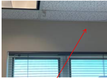
Damaged / crack in gyp. board
