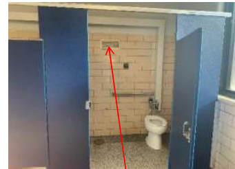
Damage to walls.
