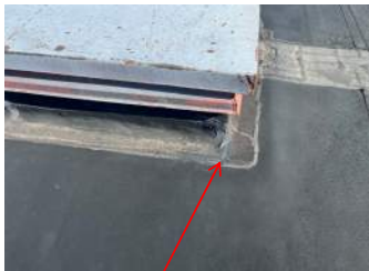
Roofing joint/seam cracking needing repair.
