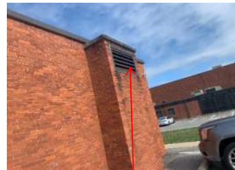
Staining at louver.
