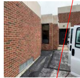
Staining on exterior wall.
