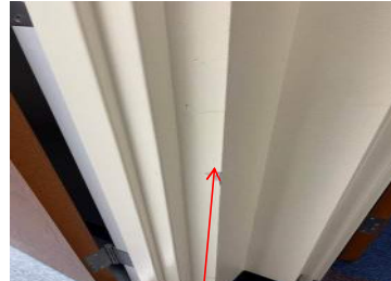
Damaged gyp. board
