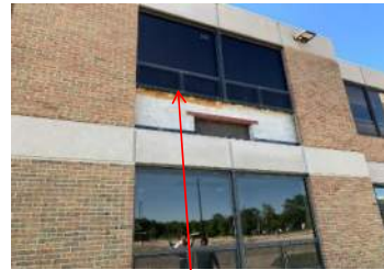
Need repairs below windows.
