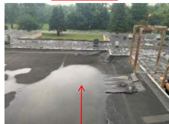
Areas of ponding.
