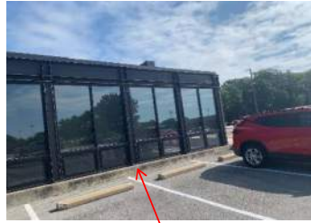
Damage at foundation - replace concrete coating.
