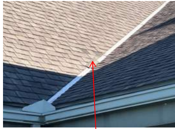
Roof shingle damage
