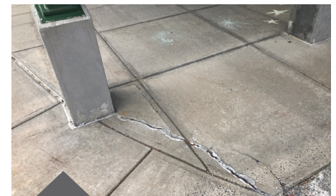
Cracked Walkways — Repairs to the radiant-heat walkway in the front of the school would be completed.
