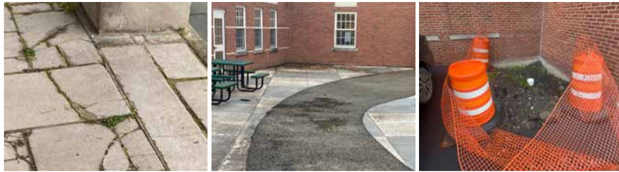
Photos of work that needs to be done
